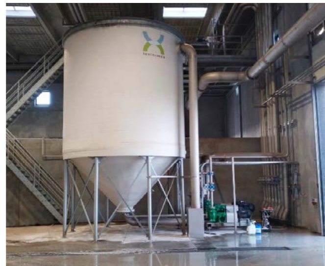
Sludge treatment facility
