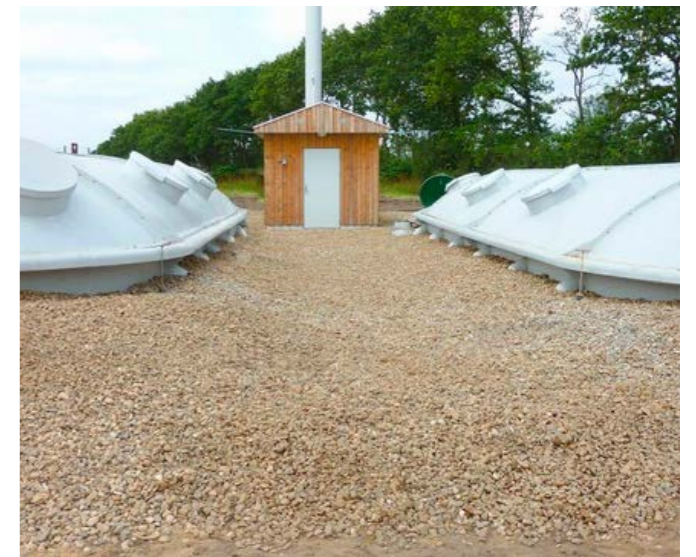
Odour and air purification facility
