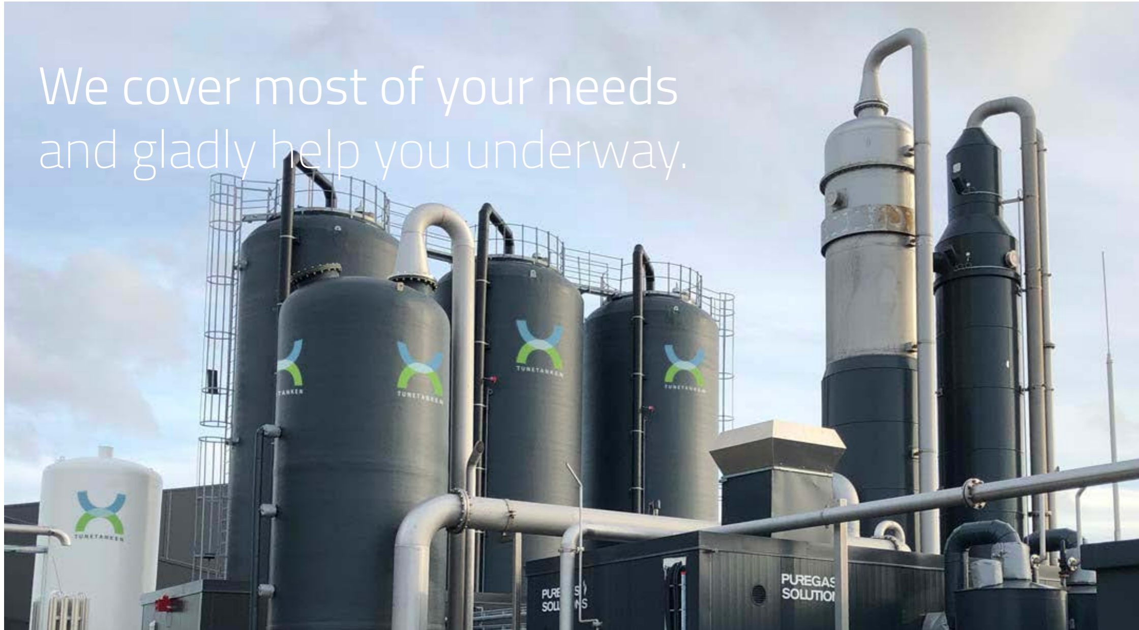
Flue gas purification facility
