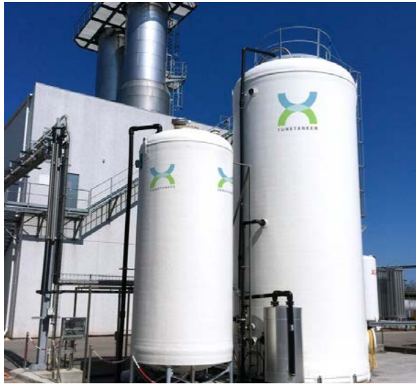
Vertical storage tanks
